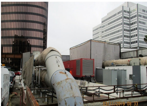
Ventilation System at Wilshire/La Cienega Station
