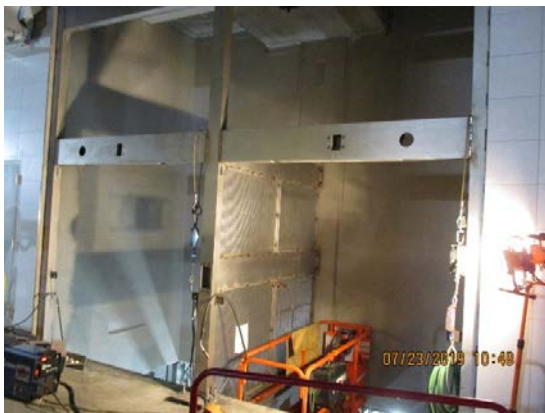
LEIMERT PARK STATION – Continued installation of elevator frames 3 and 4 at the platform level.
