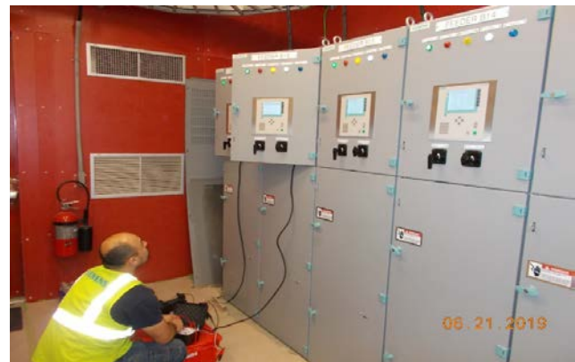
TRACTION POWER SUBSTATION #1 – Performing transfer trip test.
