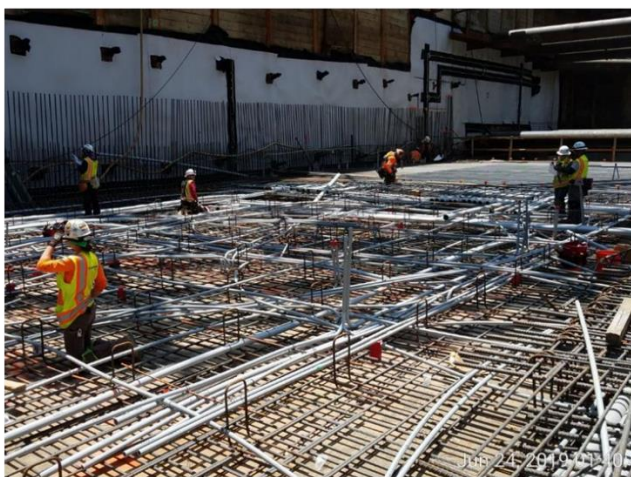
MEP conduit installation at ancillary deck level of Grand Av Arts/Bunker Hill Station
