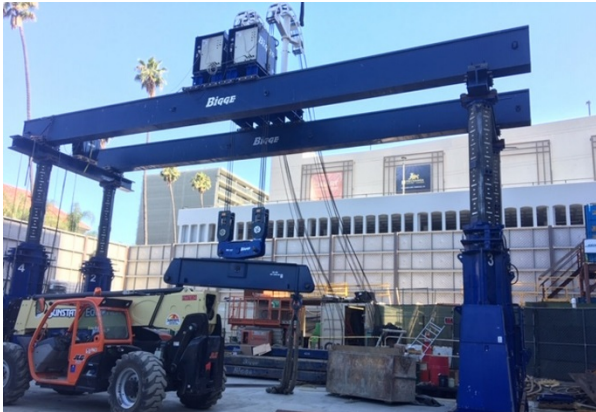
Gantry Crane at Wilshire/Western
