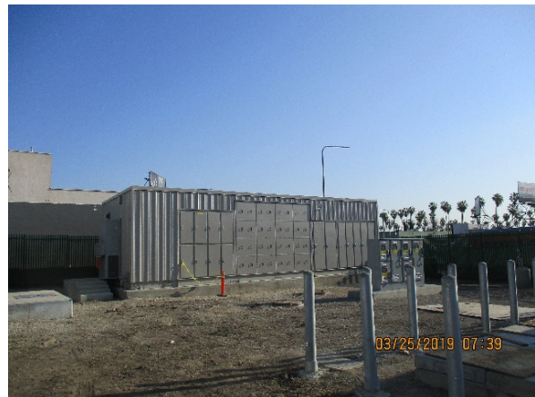
Installation of Traction Power Substation #8
