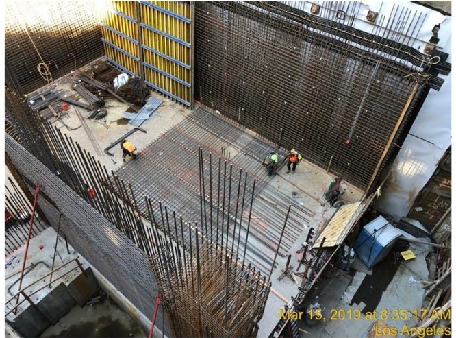
Rebar installation at interior wall at entrance structure of Historic Broadway Station
