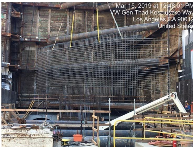
Reinforcing steel mat installation down to the Concourse Level At Grand Av Arts/Bunker Hill Station
