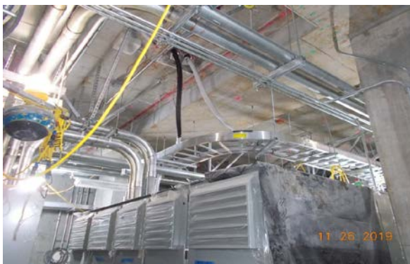
MARTIN LUTHER KING JR. STATION – Auxiliary power high voltage cable tray. 11 28 2019
