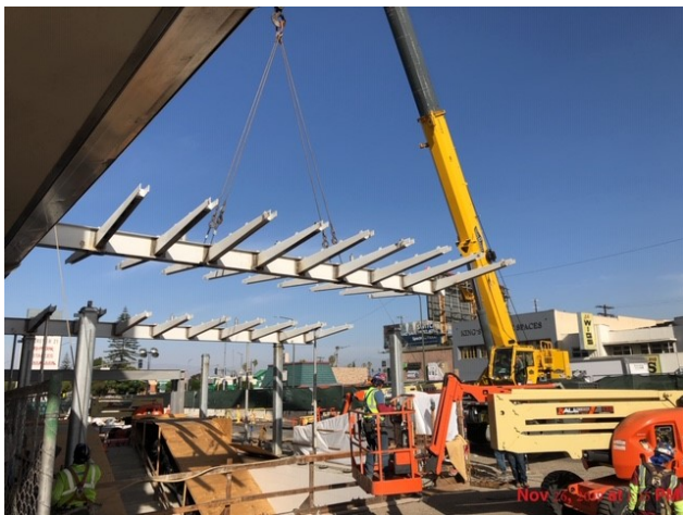
MARTIN LUTHER KING JR. STATION - Setting canopy section pieces over the main entrance of the portal. Nov 20 2019
