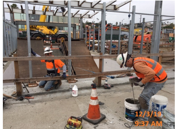
LEIMERT PARK STATION – Continued working on wind screen frames for the main entrance portal at plaza level. 12/3/19 9:37 AM
