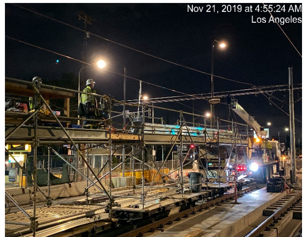
PARK MESA – Installation of overhead contact system wire from UG4 north portal to 48 th St. and Crenshaw Blvd. Nov 21, 2019 at 4:55:24 AM Los Angeles
