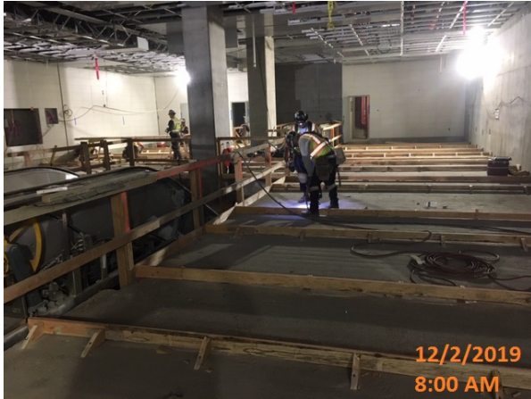
EXPO/CRENSHAW STATION – Laying and forming for architectural topping slab at concourse level. 12/2/2019 8:00 AM
