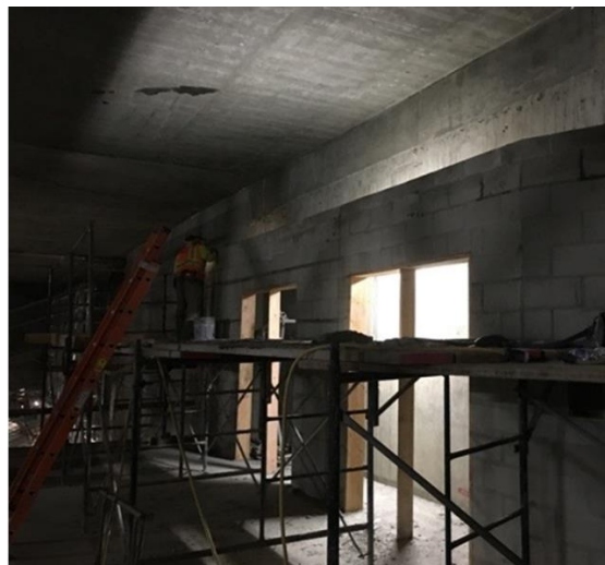
Concourse Level Escalator Control Room at Grand Av Arts/Bunker Hill Station
