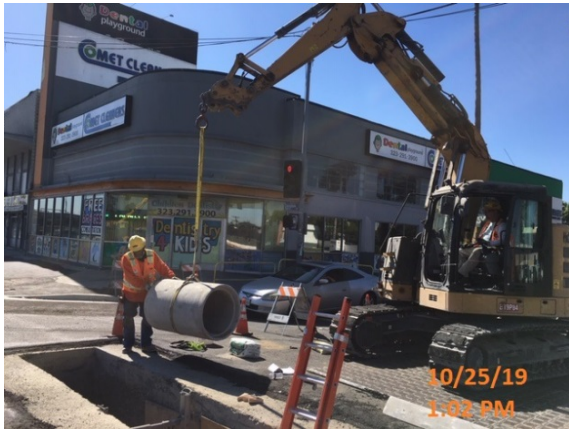
EXPO/CRENSHAW STATION – Placing reinforced concrete pipe for U – storm drain on the west side of the intersection of Obama Blvd. and Crenshaw Blvd.
