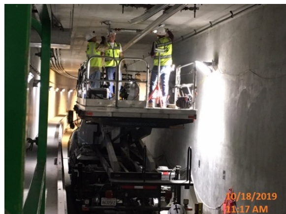
UNDERGROUND STRUCTURE #3 - Continued forms installation of overhead conductor rail for contact System on the southbound tunnel at Sta. 286 + 56.
