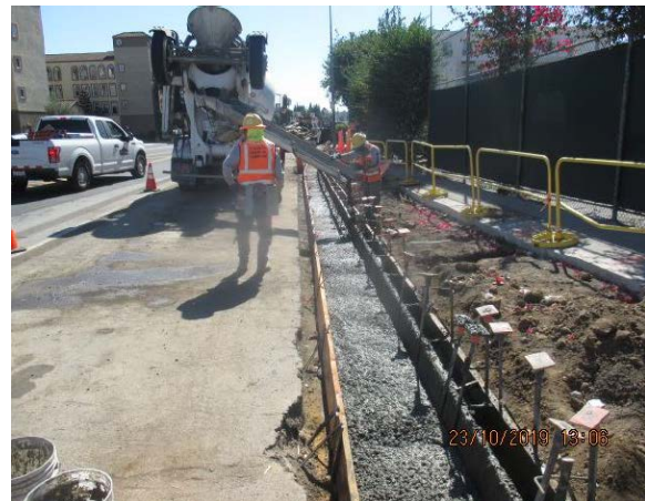
PARK MESA – Curb and gutter placement on the southbound side of 60 th St. and Crenshaw Blvd.
