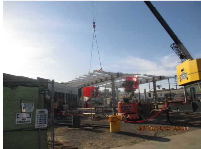
LEIMERT PARK STATION – Setting canopy piece over main entrance of the portal at the plaza level.
