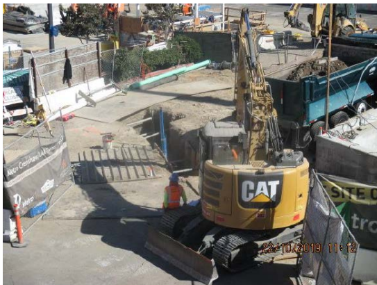
MARTIN LUTHER KING JR. STATION - Excavating Capri sewer line for E - Line. storm drain at the topside.
