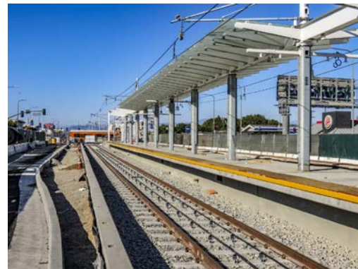
HYDE PARK STATION – Northbound view of station platform structure, completed rail, overhead power lines and landscape median.
