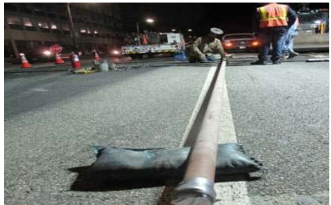
Lateral 2" Service Gas Line to be Installed on Wilshire Blvd. between Gayley Ave. and Veteran Ave.
