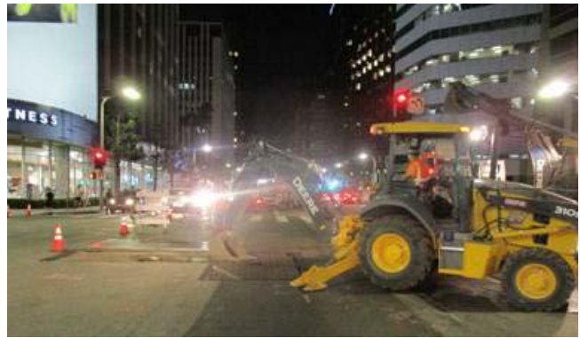
Joint Trench Excavation and Potholing for Telecom (Lateral A5) Wilshire Blvd. and Gayley Ave.
