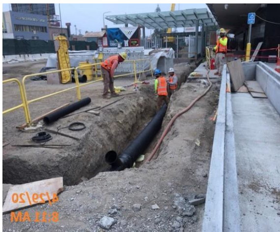
Martin Luther King, Jr. Station – Installing 12” HDPE drainage Pipe on the west side of plaza level.
