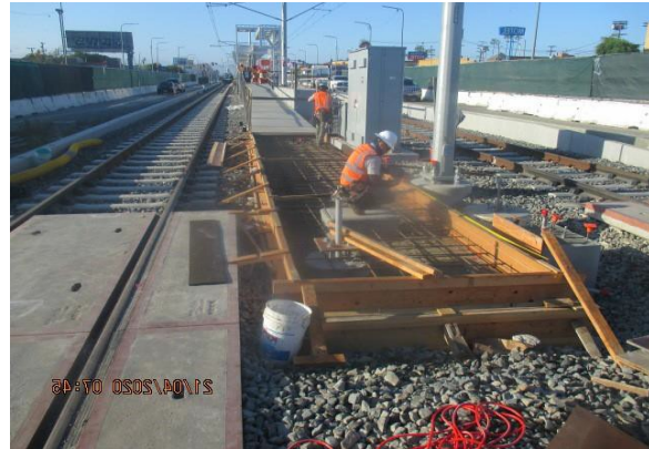
Hyde Park Station – Began formwork and rebar installation for south end entrance ramp of the platform
