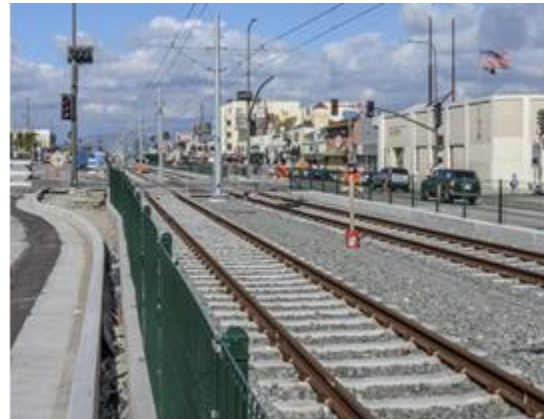
Trackwork overhead catenary system— Crenshaw and 57th Street
