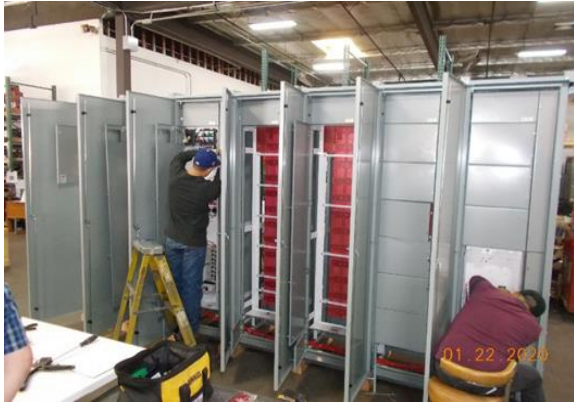
Wiring controls for testing motor control center at underground Structure No. 1
