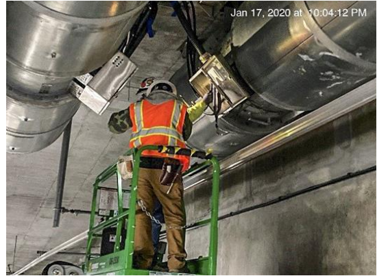
Wiring booster fans in underground structure No. 3 in the Hyde Park Area
