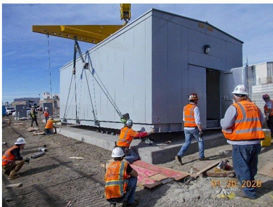
Contractor placing auxiliary power bungalow and generator at Victoria Yard in Hyde Park
