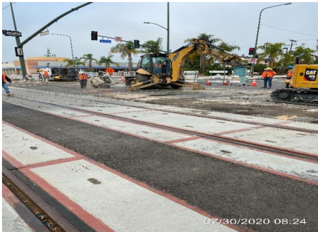
Park Mesa –Excavating/removing section of pavement southbound Crenshaw Boulevard and 54 th Street.
