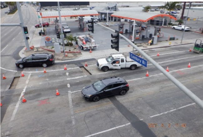
AVIATION STATION – STA 65+70 looking east – road sub-structure & surface repair (T&M); DB electric work in background
