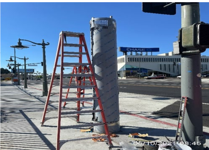
PARK MESA – Installing cover plate to the plumbing vent stack on the southeast corner of Crenshaw Blvd and 43rd Pl.
