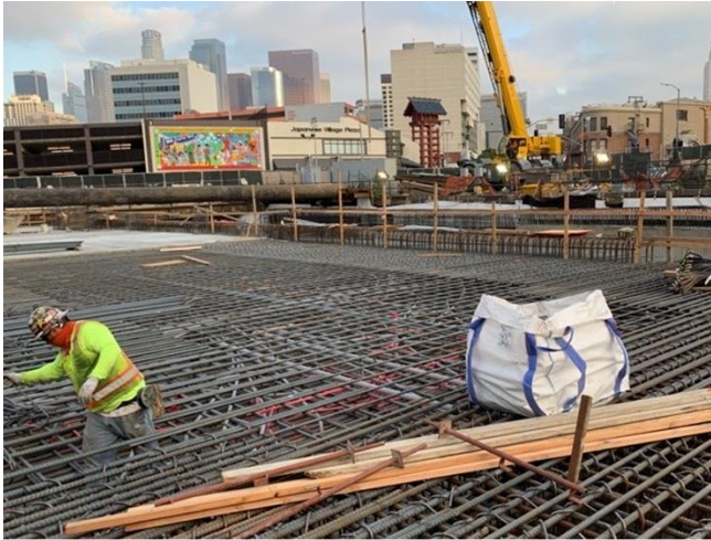
Rebar installation at roof deck at future the Little Tokyo/Arts District Station
