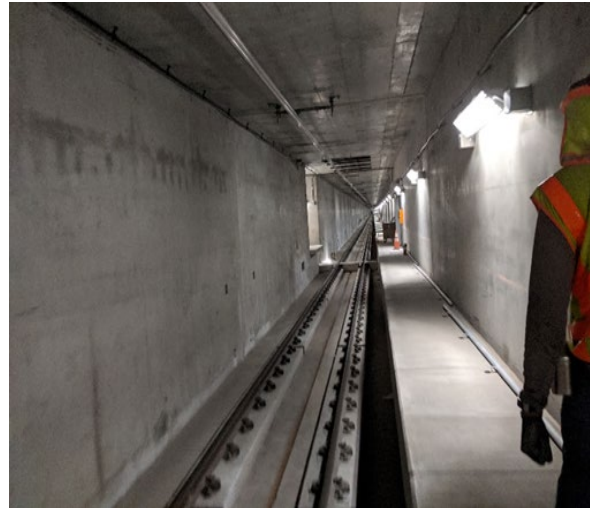
UG3 – installing galvanized handrails on north bound and south bound side of emergency walkway
