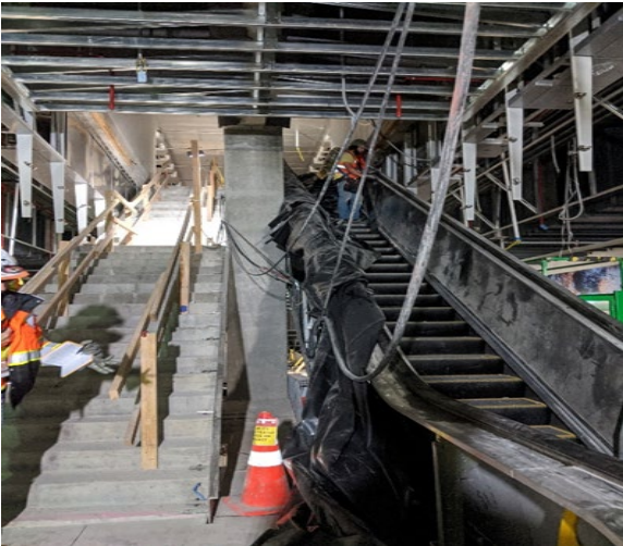
Leimert Park Station – installing stainless steel side panels Adjacent to sidewall of escalator #5
