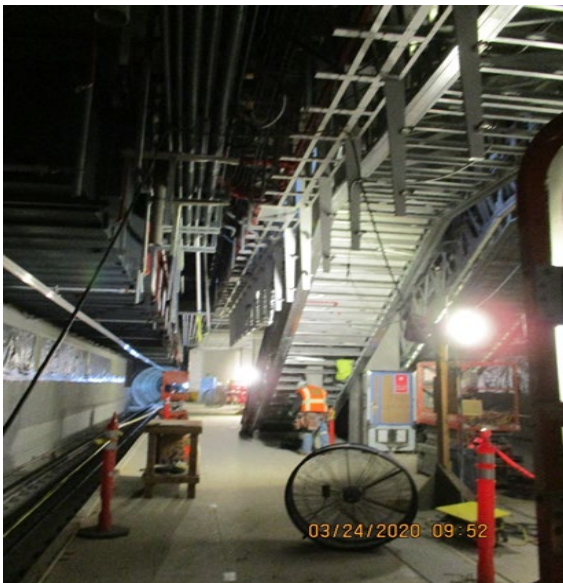
MLK Station –iron workers at north end of platform level doing layout for platform end gates on north bound side.
