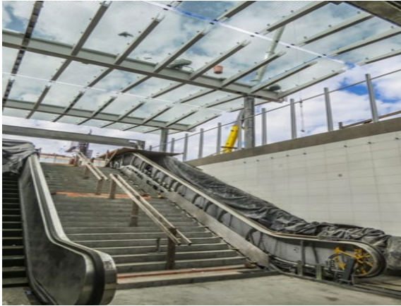
Expo Station -continuing work on interlocking double crossover breaker in TPSS room.
