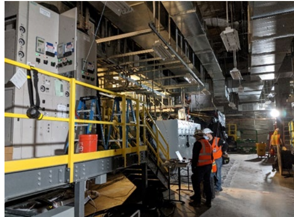
Expo Station – technicians performing testing of the main feeder
