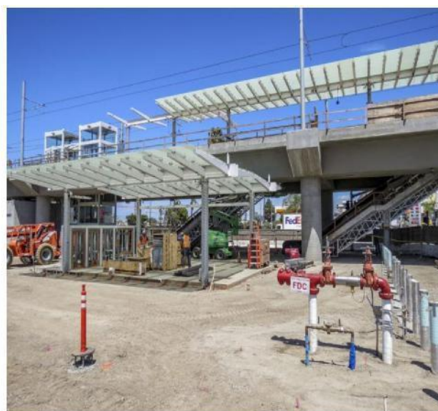
Aviation Century Station – Ticket vending machine and canopy.
