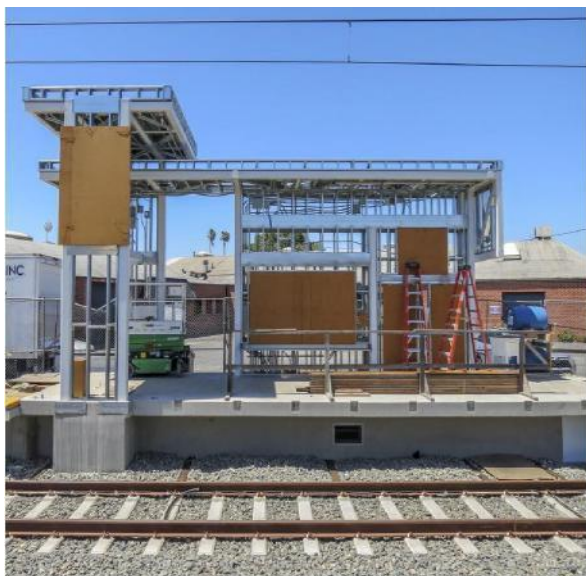
Westchester/Veterans Station – southbound station platform ticket vending machine canopy and electrical system installation in progress.
