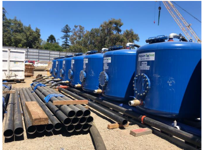
Dewatering Resin Filters at VA
