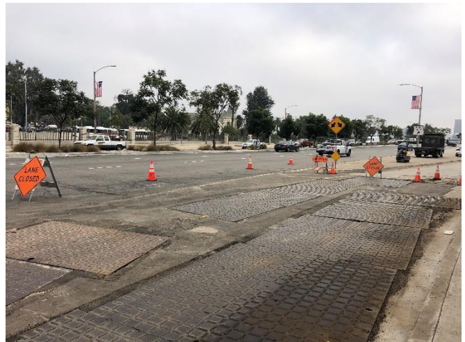
Installation of SCE Duct Bank & Substructure along Wilshire to Bonsall Entrance Ramp near VA
