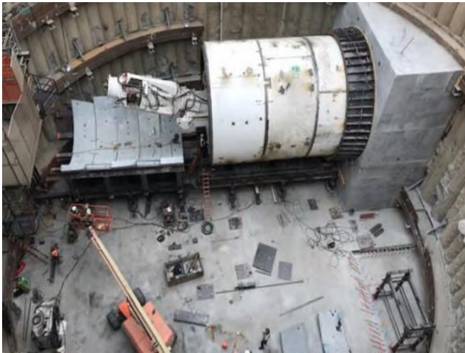
Installation of Temporary Invert Segments on Gantry Cradle at Base of Excavated Tail Track Exit Shaft
