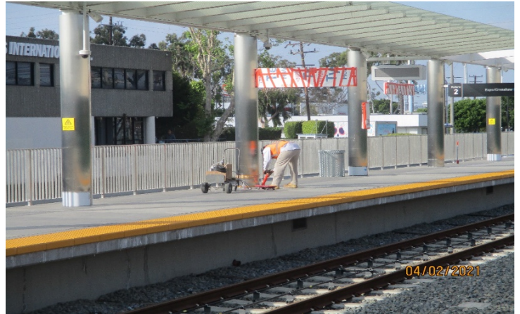
HINDRY STATION – Placing sealer caulking for the Hindry Station Columns (facing southwest).
