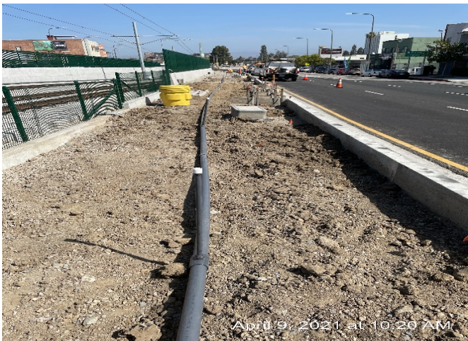
PARK MESA – installing irrigation lines along the northbound median of Crenshaw Blvd. between 48 th St. and 46 th St.
