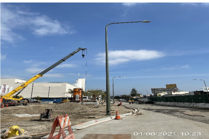
MLK STATION – Installing street light poles along the east side of the far south section of the plaza.
