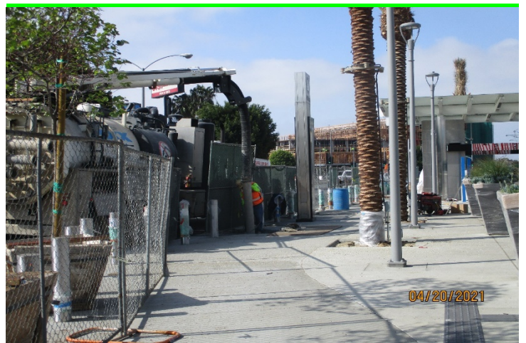
LA BREA STATION –Excavating for the trees at the La Brea Plaza (facing west).
