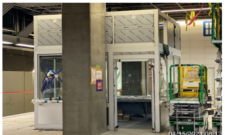
EXPO STATION – Continue assembling the Supervisor Room at the south end of the platform
