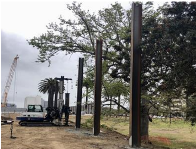
Installation of Sound Barrier Wall Piles at Westwood/VA Station – West of Bonsall
