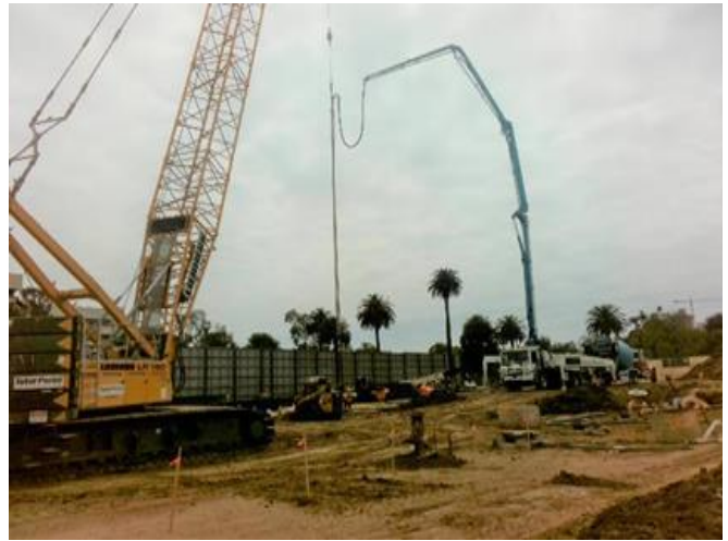
Concrete Pour in Process for Installation of Support of Excavation Soldier Piles at Westwood/VA Station
