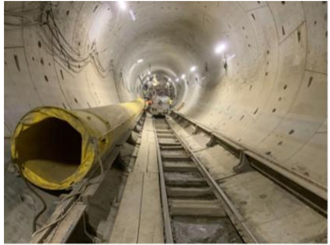
Temporary Ventilation System for "Aura" TBM
