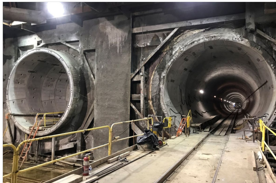
Wilshire/Western Interface Chamber
