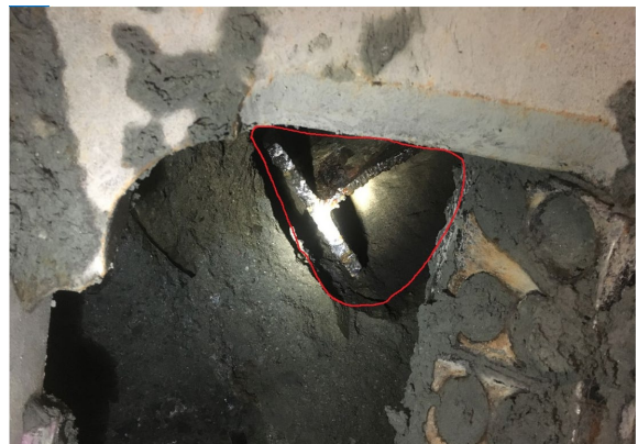
I Beam (Anomaly) Discovered in North Tunnel
