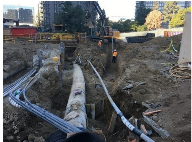
Excavation for temp relocation of 24" storm drain bypass at Historic Broadway Station
