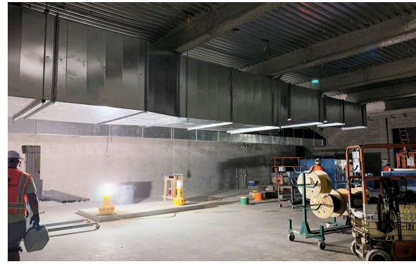
Concourse HVAC Ductwork at Wilshire/La Brea Station
