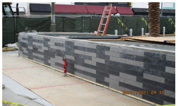
MLK STATION – Continue granite tile installation to the exterior walls of the Fresh Air Intake Shaft 2.
