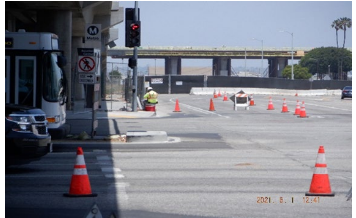
AVIATION/CENTURY STATION – STA 68+50 looking north – Aviation/Century Street lighting work by DB Electric
