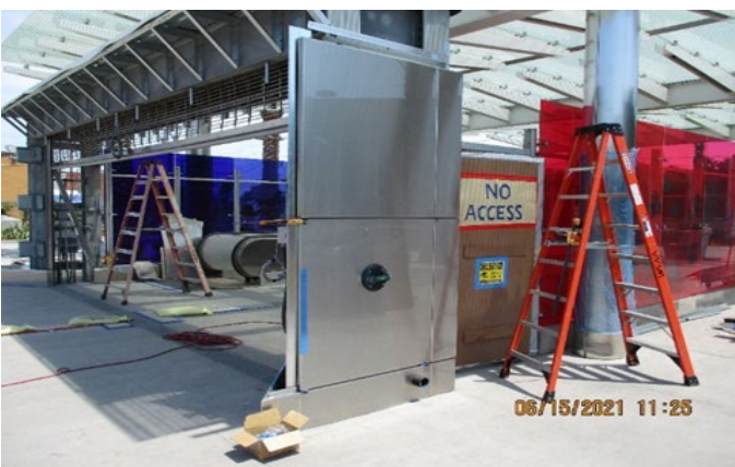
LEIMERT PARK STATION – Continue cladding installation to the main entrance coiling door at the plaza.
