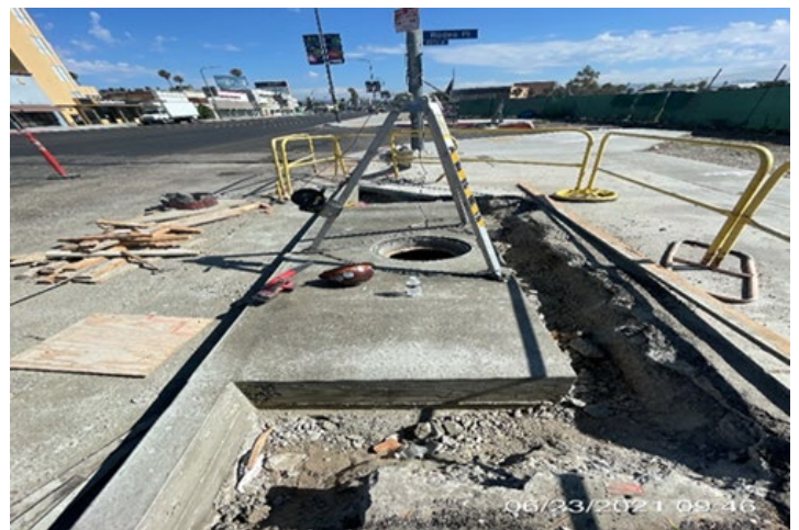
EXPO STATION SITE – Removing formwork from Catch Basin #11 on northbound Crenshaw Blvd and Rodeo Pl.
