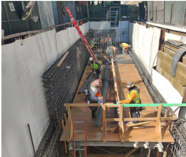
West vent walls and upper deck formwork and rebar at Historic Broadway Station
