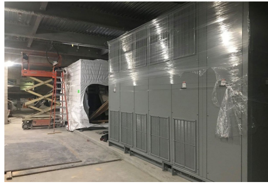
Transformer Placement at Wilshire/La Brea Station
