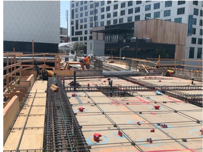
PVC and device boxes in Ped Bridge Pavilion Deck of Grand Av Arts/Bunker Hill Station
