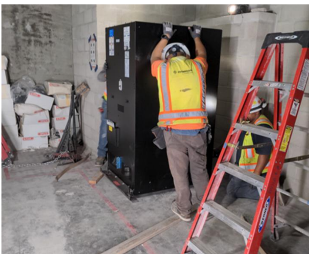
Battery cabinet installation in the TC&C battery room at Little Tokyo/Arts District Station
