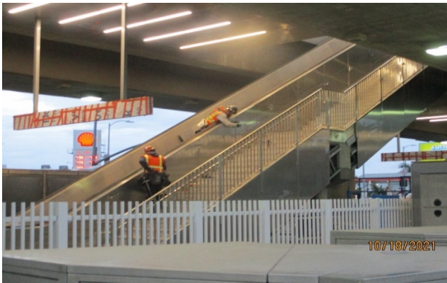
AVIATION STATION – Mounting the stainless steel cladding panels at the Aviation Station Plaza
