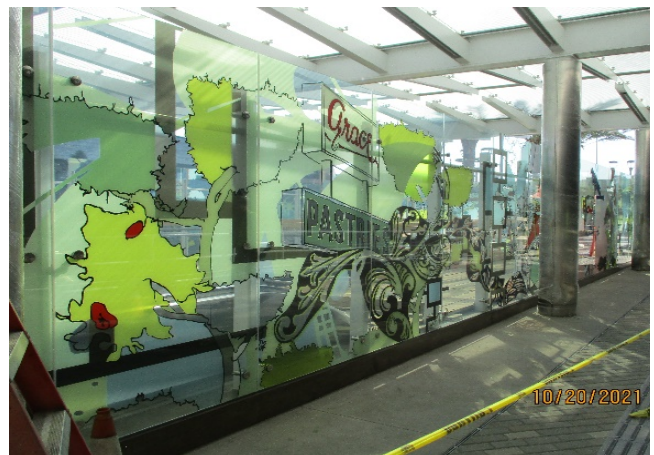
MLK STATION – Continue art glass panel installation around the perimeter of the main entrance plaza canopy.
