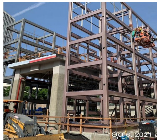
Welding for hoist way frames at PL3-6 at Grand Av Arts/Bunker Hill Station
