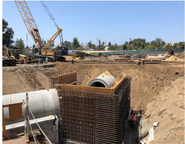
VA Steam Tunnel Section Backfilled to Allow Crane Transfer to Bonsall Ave
