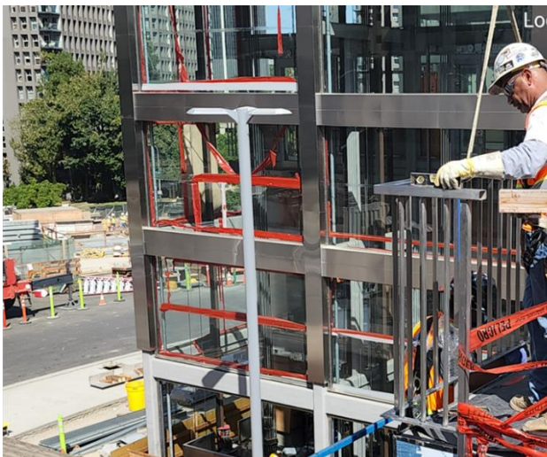
Handrail installation at Upper Plaza Level at Grand Av Arts/Bunker Hill Station
