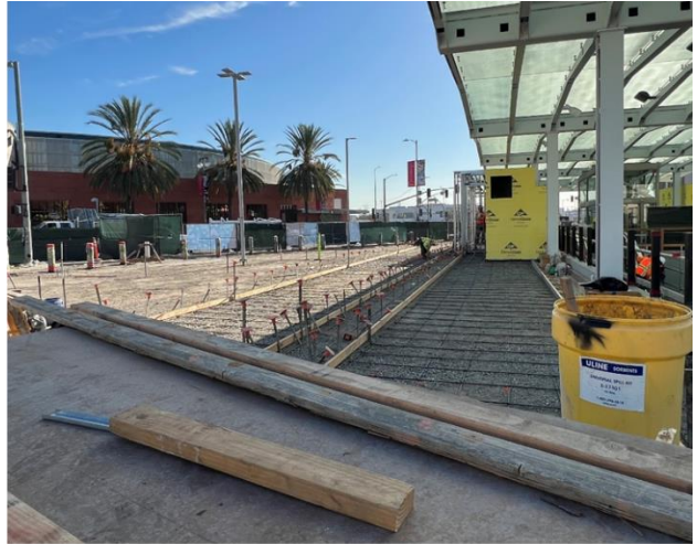
Foundation at east corner of Entrance level at Little Tokyo/Arts District Station
