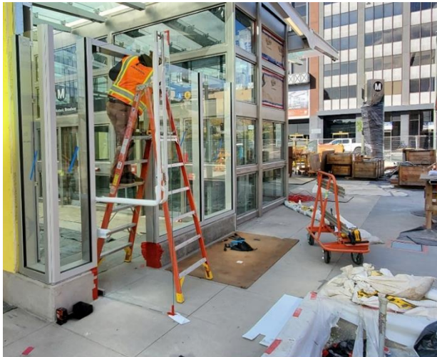
Installation of glass exit door at north Plaza at Historic Broadway Station
