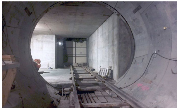
Wilshire/Western Interface Chamber Box Structure
