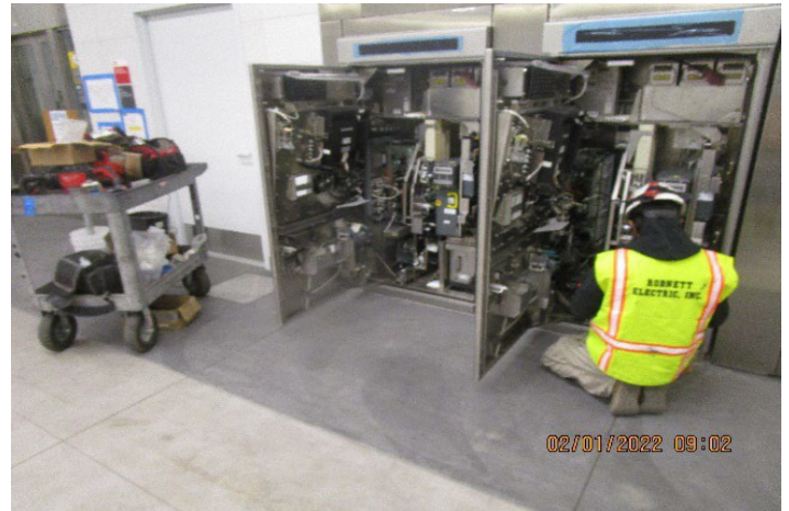
LEIMERT PARK STATION – Energized and performed integral verification testing of the ticket vending machines and fare gate system at the Paid & Free Area.
