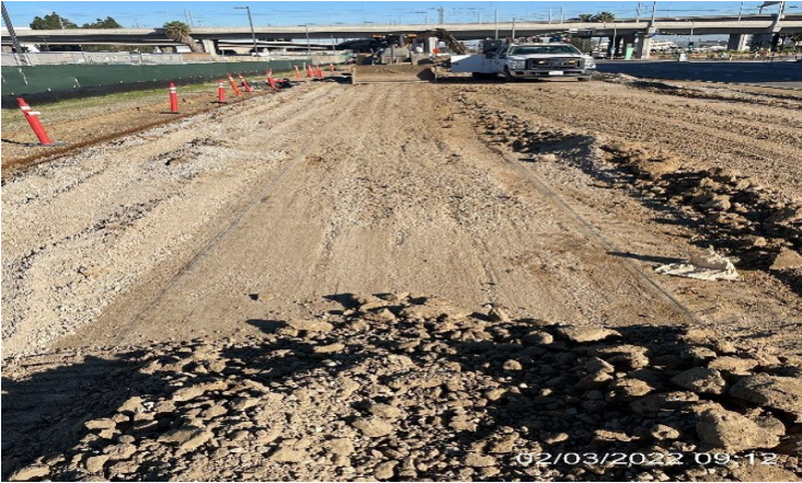
AVIATION STATION – WSCC exposing top of rail at Aviation and 118th street
