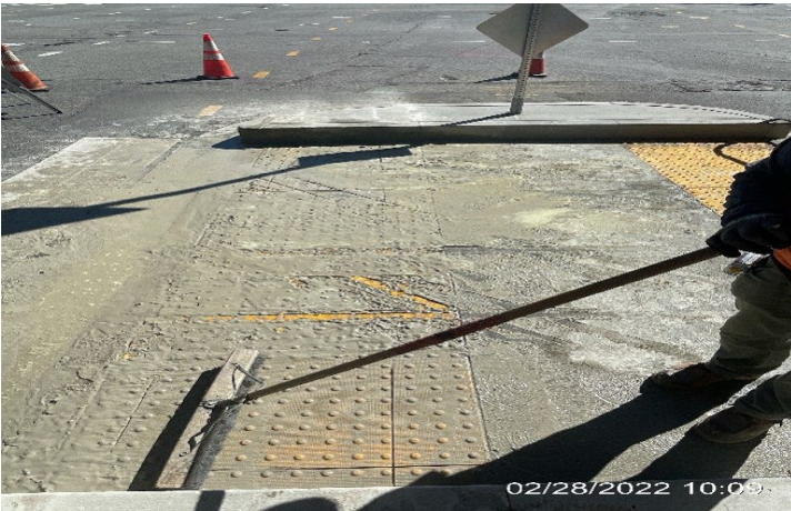
CENTURY STATION – WSCC saw cutting dome at ADA Ramp located at Century Aviation.
