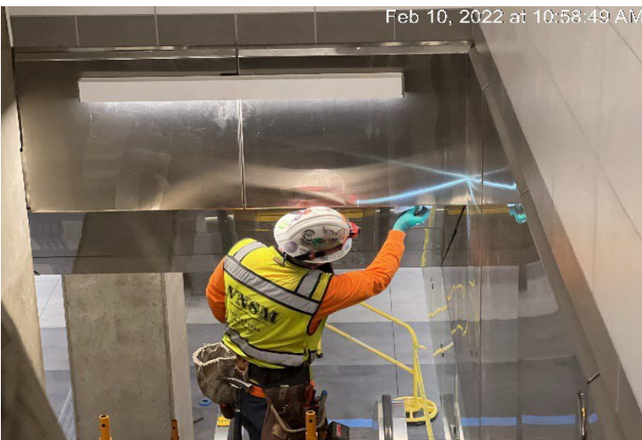
MLK STATION – Adjusting stainless steel cladding panels above Staircase 3 at the concourse.
