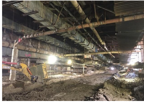
Excavation and Utility Support Activities West of the Launch Box in Century City
