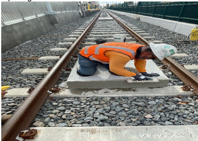
HYDE PARK STATION – Sacking and patching light rail vehicle pads along the southbound track near Slauson Ave.
