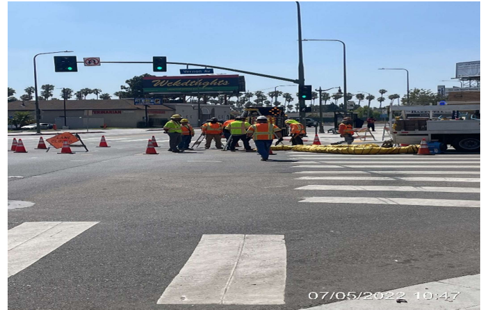
LEIMERT PARK STATION – Inspecting the sewer line along southbound Crenshaw Blvd and Vernon Ave.
