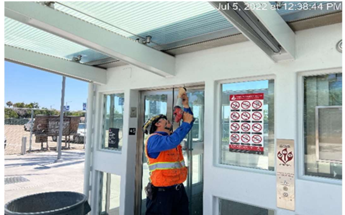
EXPO STATION – Applying caulking around the door openings of Elevators 1&2 at the plaza.
