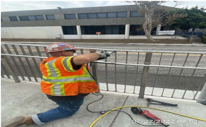
HINDRY STATION – WSCC making corrections to the iron fencing at Hindry Station.
