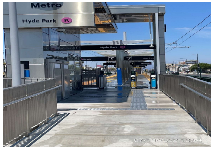
HYDE PARK STATION – Performing water leakage test to verify water does not intrude inside the TC&C Room.
