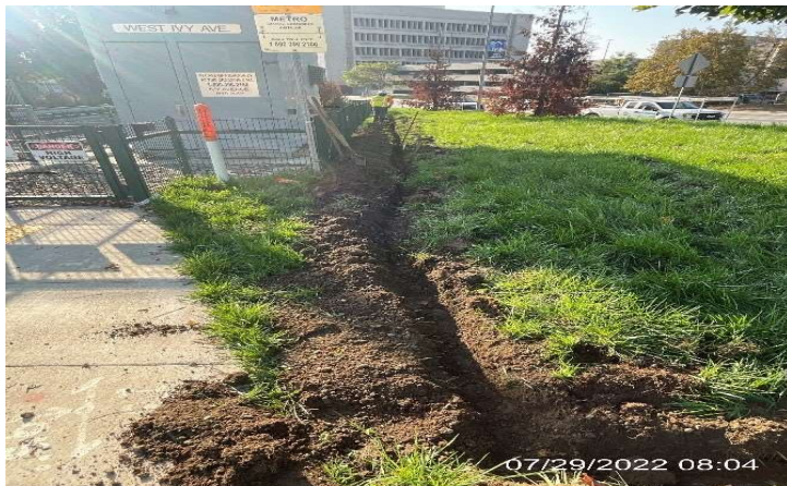
CRENSHAW - Marina trenching to install irrigation line at Florence and Ivy, WB Florence.
