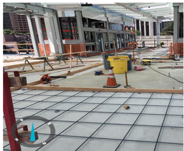
Formwork and rebar at Upper Plaza Pavilion at Grand Av Arts/Bunker Hill Station
