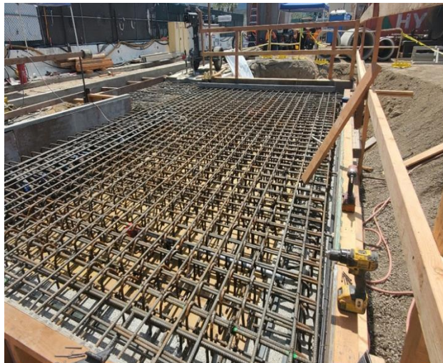
Rebar and forms installation at the ES3 shaft roof slab at Historic Broadway Station
