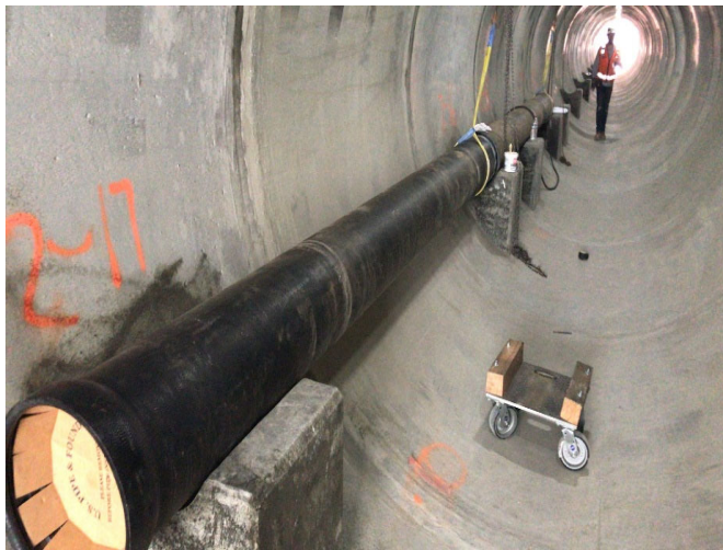
Westwood/VA Station Installation of 12-in Ductile Iron Waterline Inside the VA Steam Tunnel
