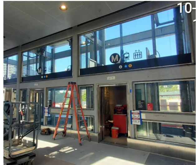
Installation of station signage on PL1-PL3 elevator tower at Grand Av Arts/Bunker Hill Station
