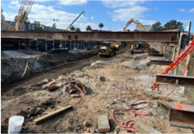
Excavation of Westwood VA Station Box to Level 1 Bracing, East of Bonsall
