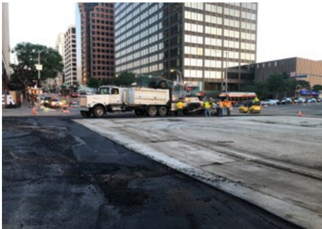
Westwood/UCLA Station Facing East – Street decking and paving at Wilshire and Westwood
