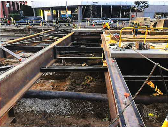
Westwood/UCLA Station Facing South Install & Weld Cross Braces, Laterals, and Deck Beams
