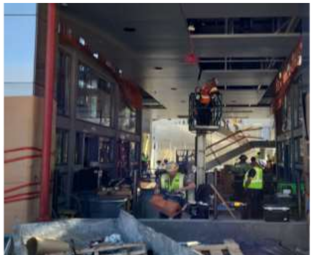
Installation of fire alarm at Grand Av Arts/Bunker Hill Station Plaza Level
